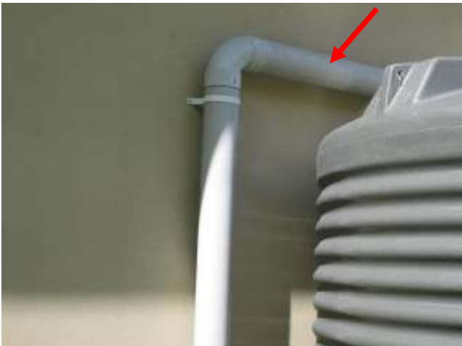
Incomplete paint finish to external PVC water tank pipes
