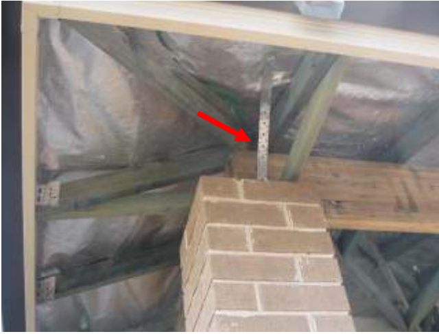
Hoop iron strapping must be fixed as intended to roof pitching beams
