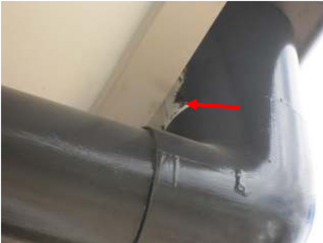
Incomplete paint finish to external PVC downpipes
