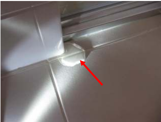
Leaking showers after the flood testing
