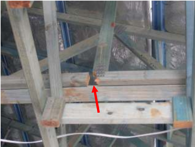
Rectify broken or damaged roof truss tension bracing and or bottom chords
