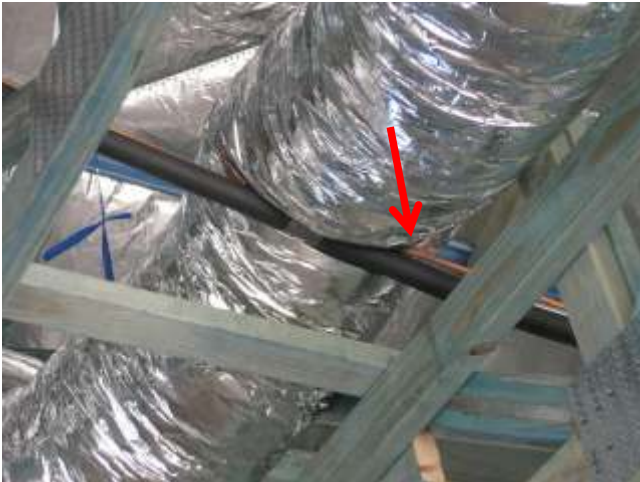
Bare copper pipes must not be in contact with A/C ducting materials
