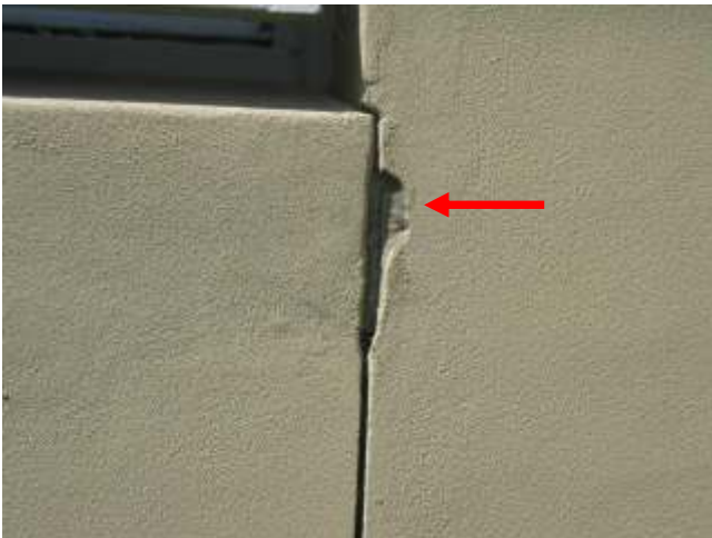
Chipped render to external walls
