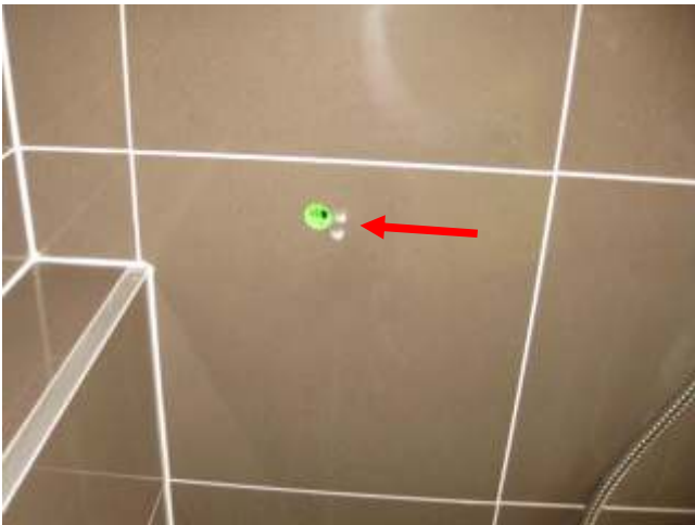
Incomplete wall tile replacement due to poorly fitted PC items!
