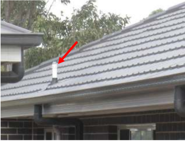
Incomplete paint finish to the roof top PVC sewer vents pipes
