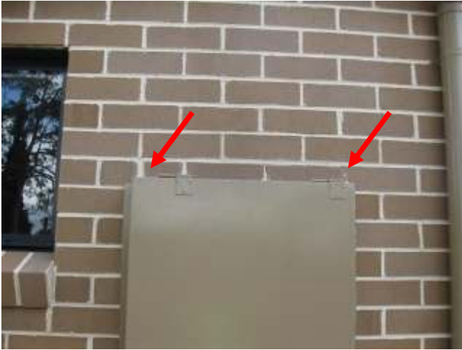
Incomplete brickwork and non-compliance
