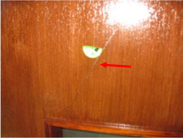
Scratched stain finish to doors
