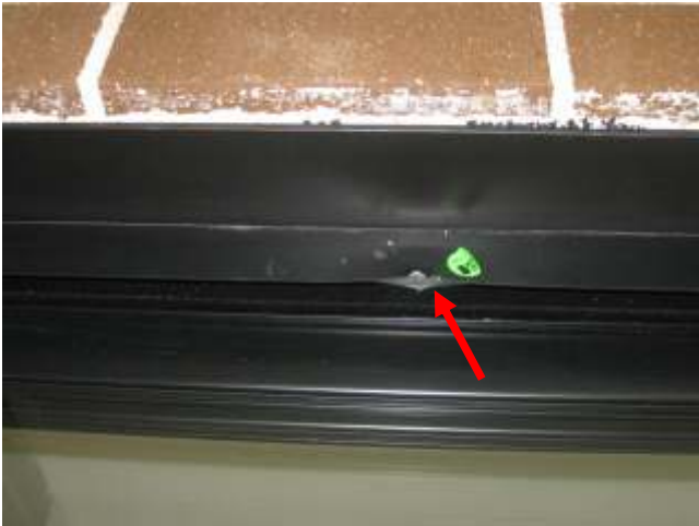
Damaged aluminium door and or window frames
