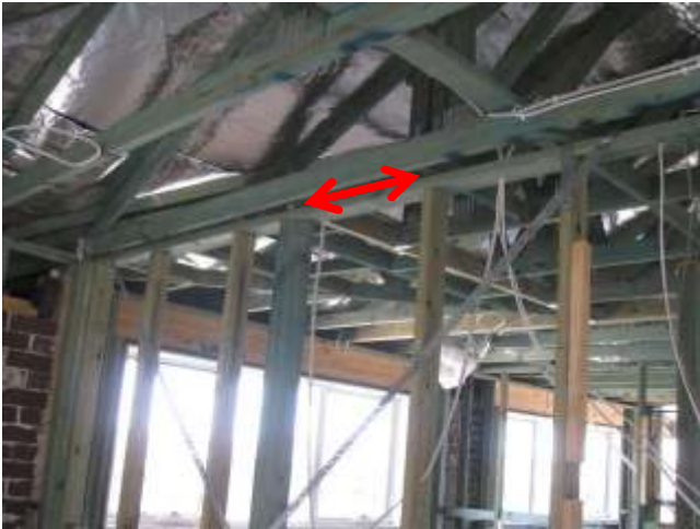
Shear blocking incomplete above internal braced walls
