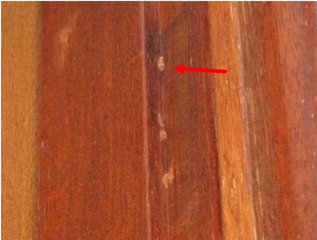
Incomplete paint finish to external door jambs
