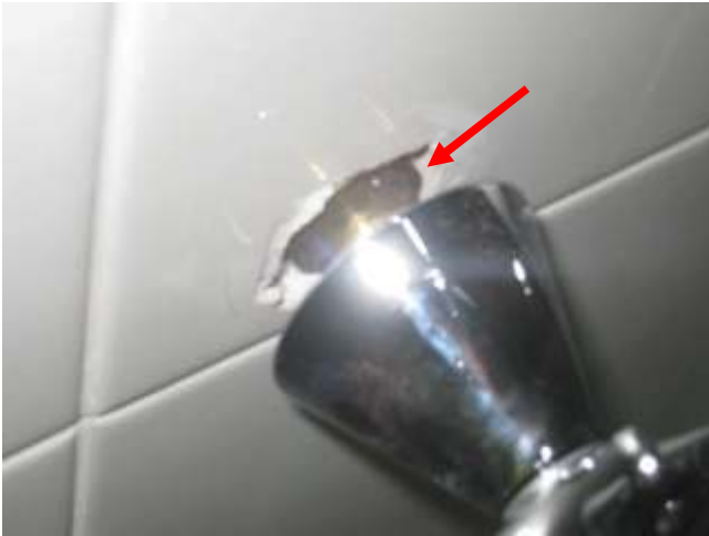
Shower Taps NOT sealed
