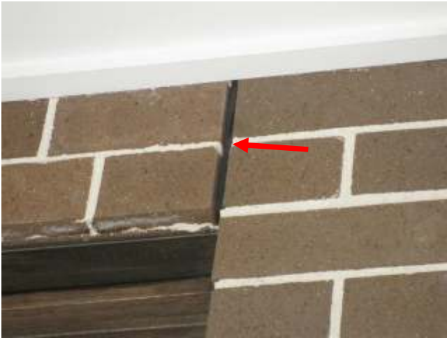
Incomplete mastic seal to brick expansion joints
