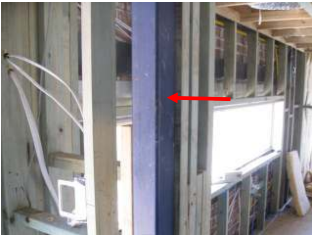
Incomplete wall studding to the external corner areas of steel columns
