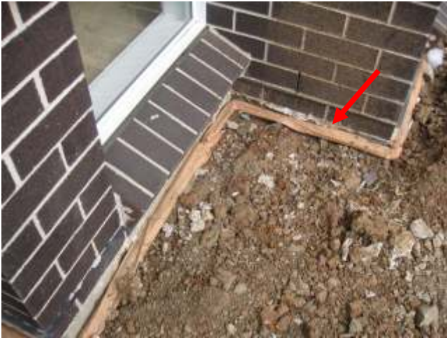
Termite Barriers yet to be covered and charged up as intended
