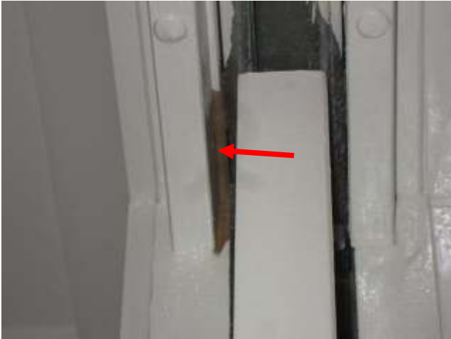
Incomplete paint finishes to the interiors of cavity door pelmets
