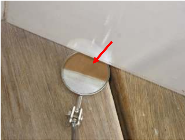
Undersides and top edges of external and wet areas doors are not sealed as intended
