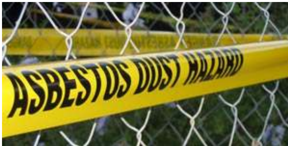
Signage must be used when removing Asbestos
