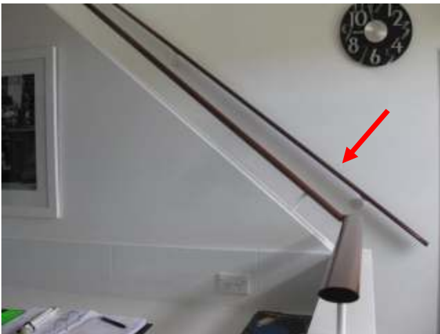
Stairwell railings out of parallel
