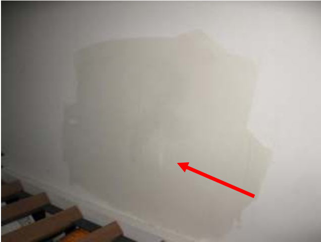
Incomplete plasterboard setting, sanding and paint finish
