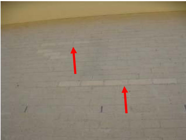
Wrong coloured brick installation
