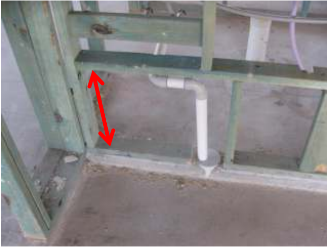
Stud trimming incomplete under frame alterations
