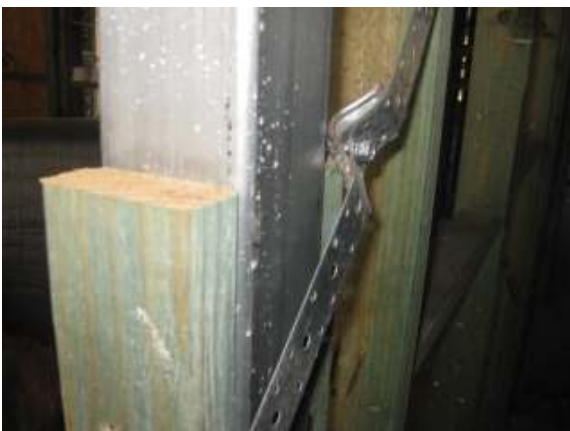
Wall bracing fouled by steel columns
