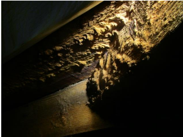
Damaged roof timbers
