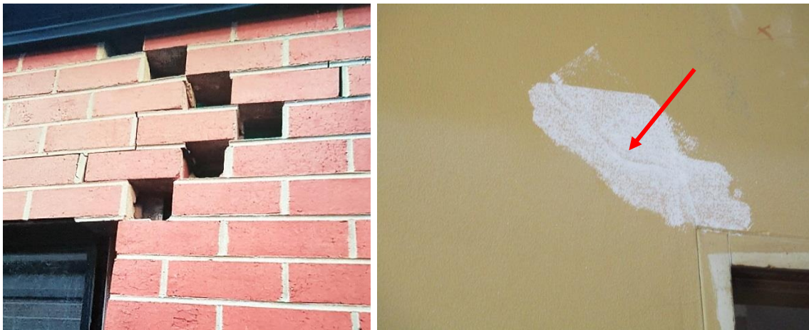
Excessive movement and internal wall cracking
